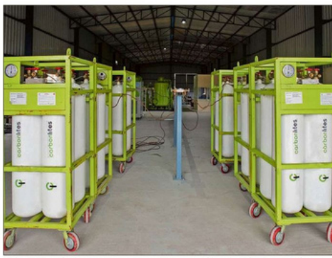
Bio-CNG cylinders at the wet waste processing plant in Harohalli PHOTO/SPECIAL ARRANGEMENT
