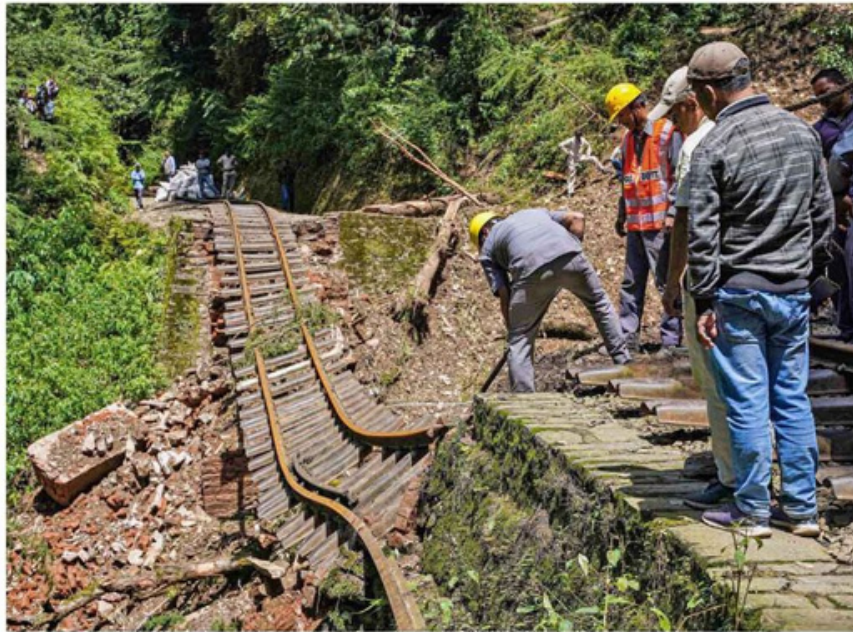
Wrath of the skies: The Kalka-Shimla railway track after it was damaged due to a landslide following heavy rainfall in Shimla on August 26. PTI
